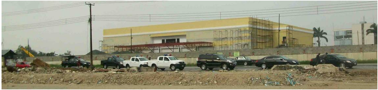
Silverbird Showtime under construction (12 March 2009); in the foreground, the rubble of buildings demolished (10-13 February 2009) to make way for a parking area © J. Falade
