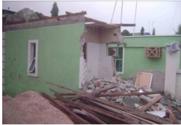
A wall that had encroached on the road reserve in GRA is marked for demolition © R. Precht
