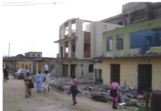
Demolished legal structures in Nanka Street; New Niger Hospital (under construction) in the background © R. Precht
