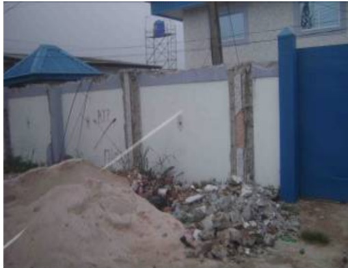
Partly demolished “illegal structures” that were erected beyond a plot boundary in GRA © R. Precht
