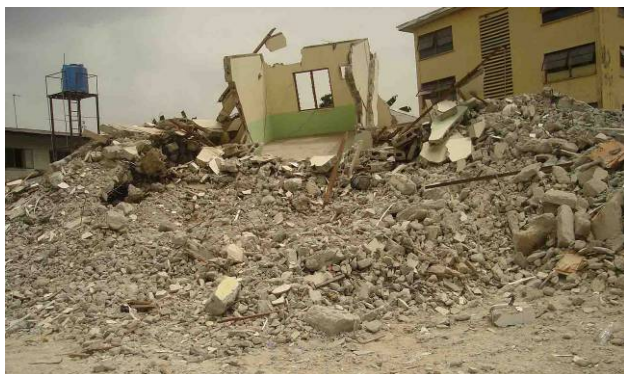
Half demolished legal buildings on Abonnema Wharf Road, during demolitions 10-13 February 2009 © SERAC
